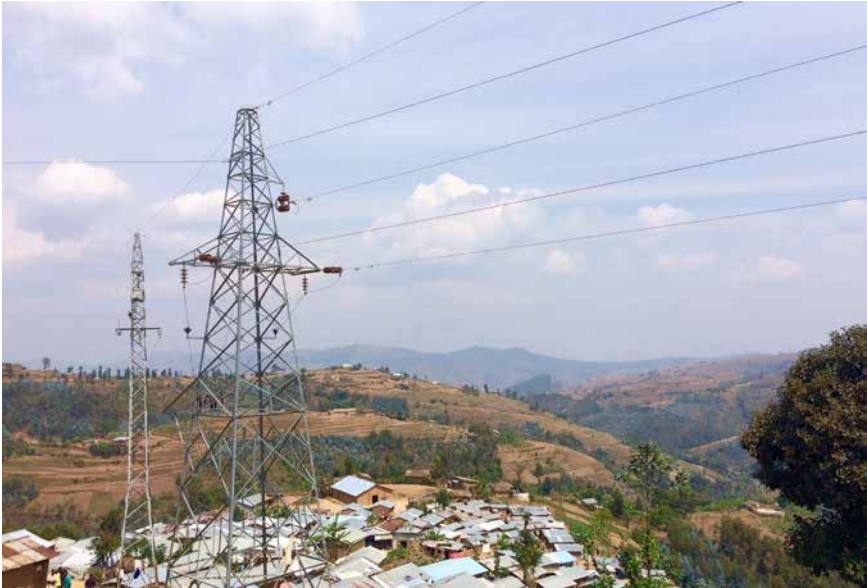
Figure 3.5. Electricity connections overhead in Kigeme, Rwanda. © Sarah Rosenberg-Jansen.
